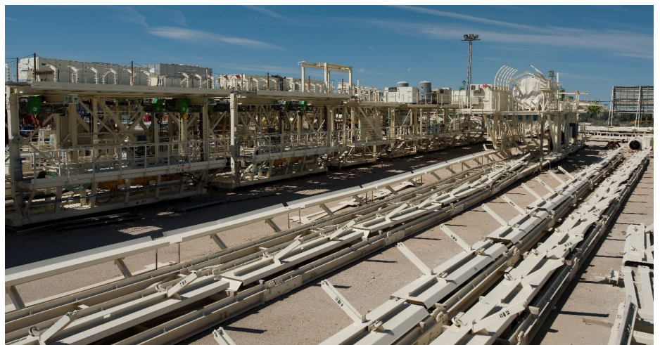
Close up of a TBM
